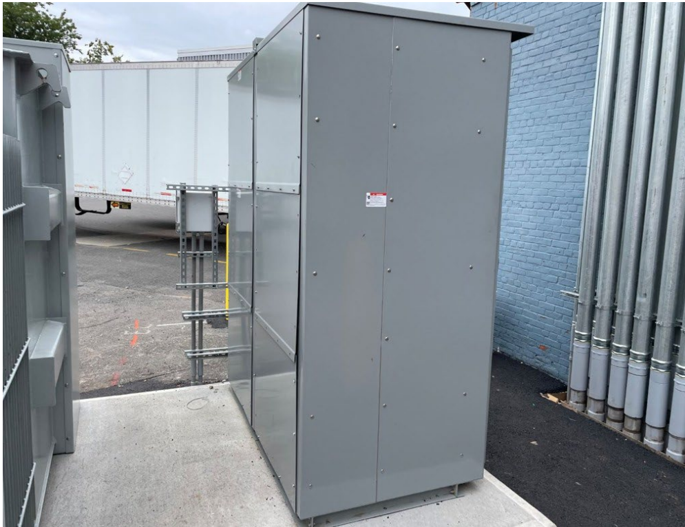
Figure 6: Equipment example: Switchgear
