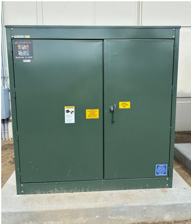
Figure 5: Equipment example: Transformer
