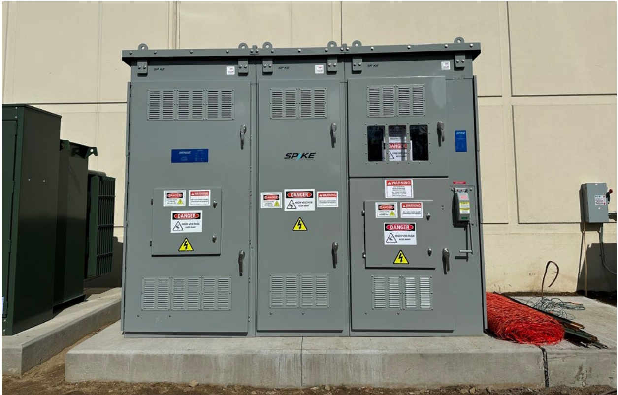
Figure 4: Equipment example: MV Disconnect
