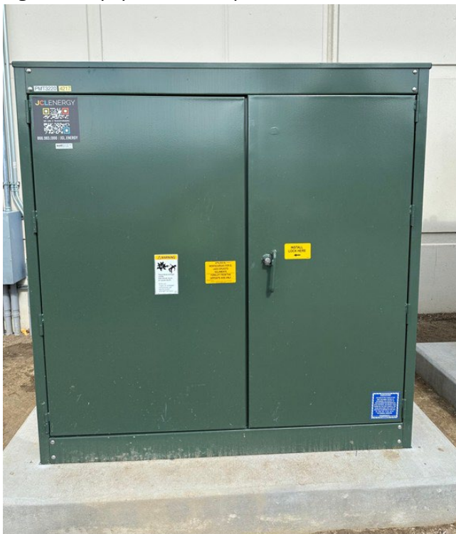
Figure 5: Equipment example: Transformer
