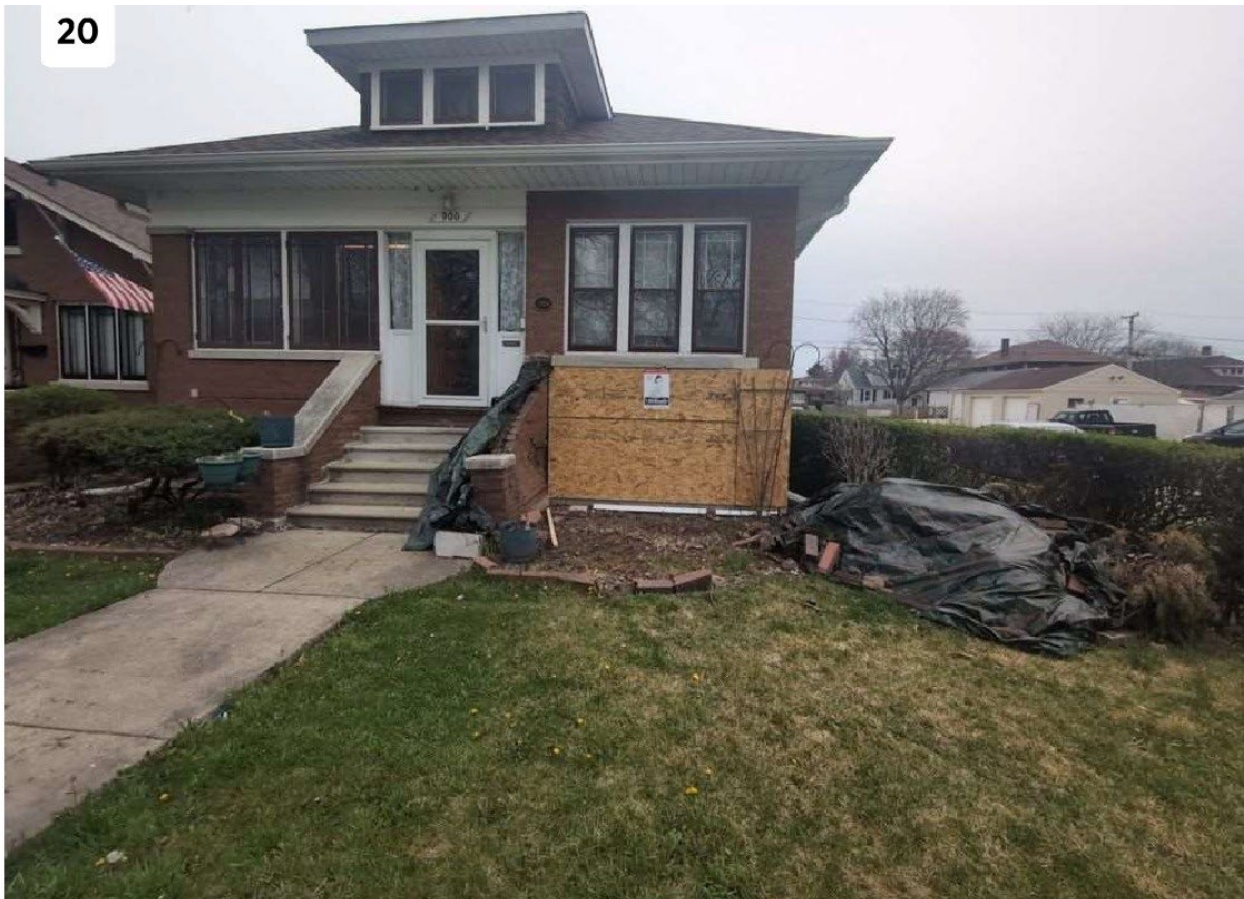
House in April 2024, showing the damage to the front façade
