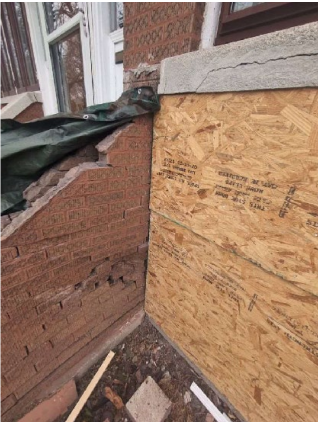
House in April 2024, showing the damage to the front façade
