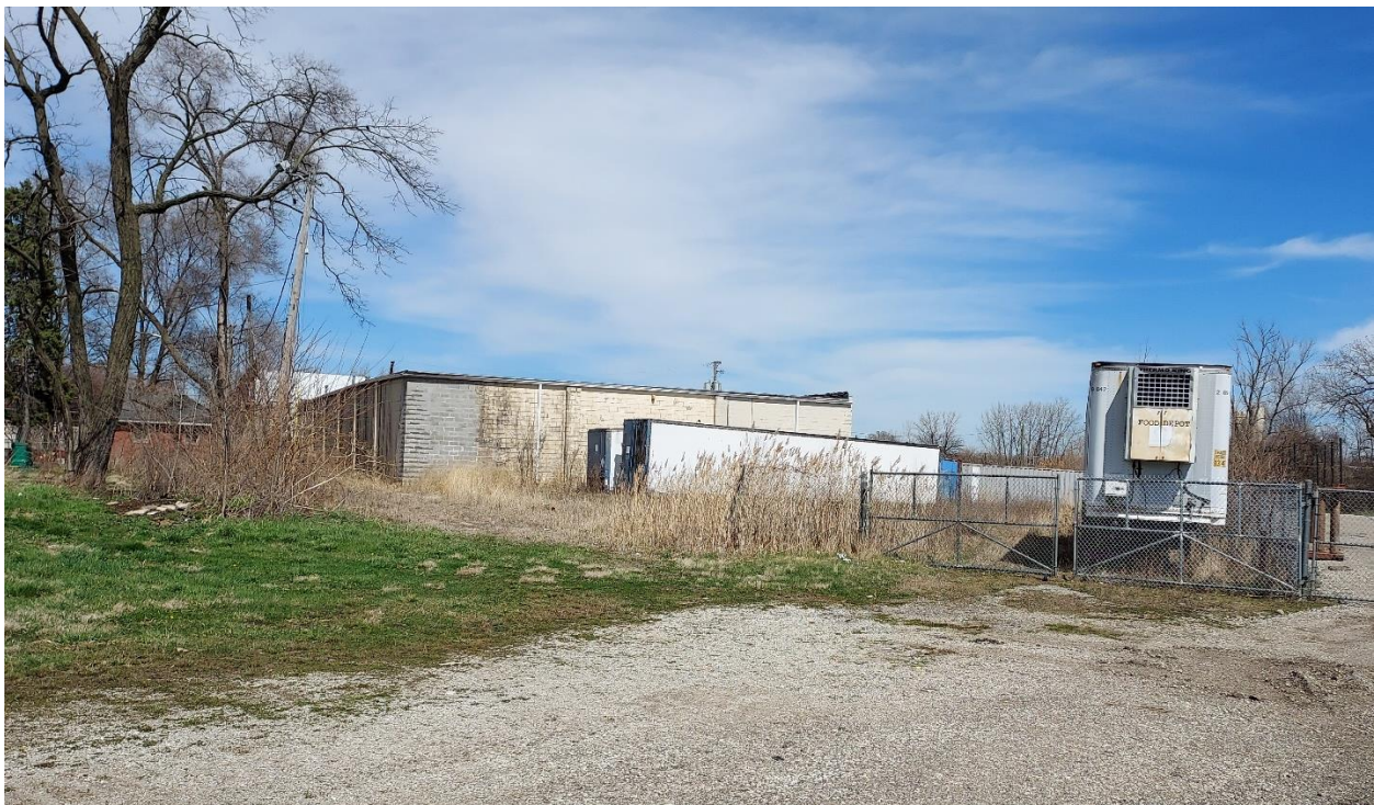
Figure 4: Existing concrete block building – proposed to be remodeled for climate-controlled indoor storage
